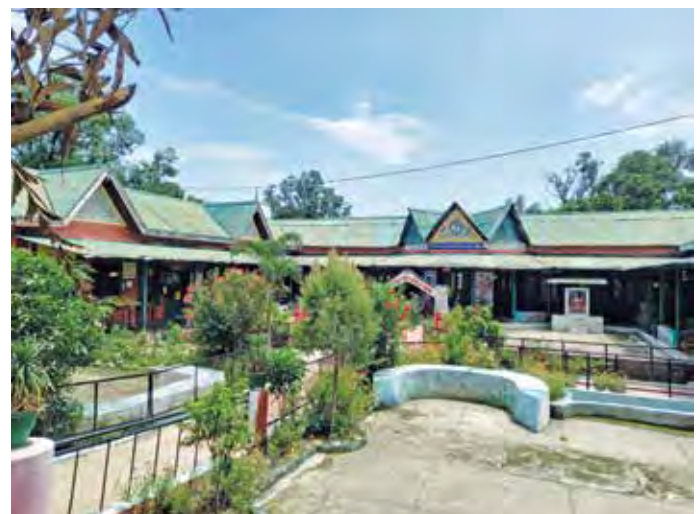
Figure 5: Gable roof with corrugated metal sheets at Govt. Girls School in Garli Source: Author
