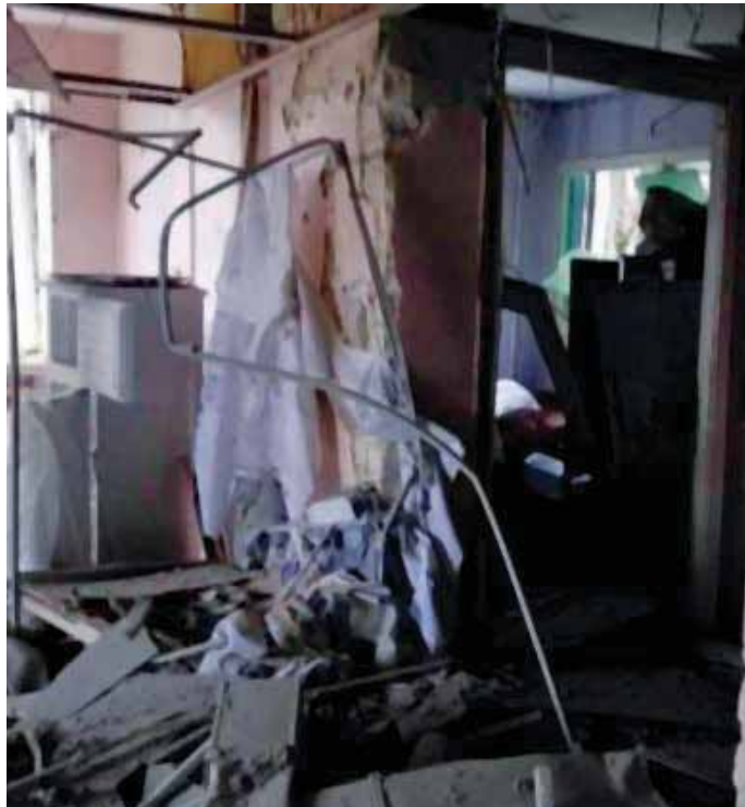
Fig.5: Damage to the Vasylivka Multidisciplinary Intensive Care Hospital. (Source: Retrieved, January 15,2023 from https://www.directrelief.org/ )
