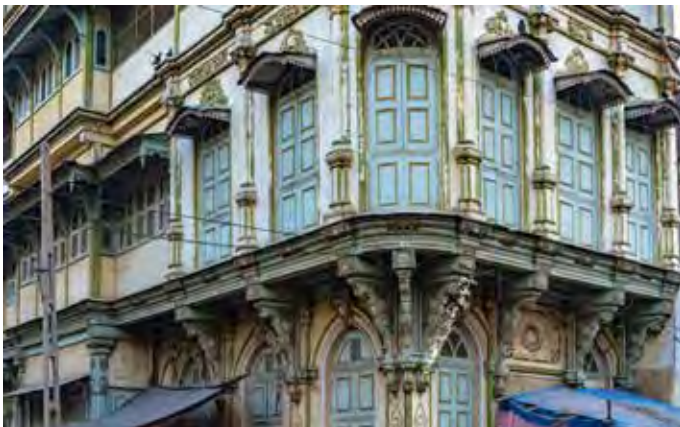
The other face becomes clearer, and you can notice it being present on the buildings themselves, their age and decay starkly visible if you took a closer look.
