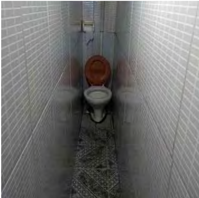
Figure 8: Narrow space to access WC
