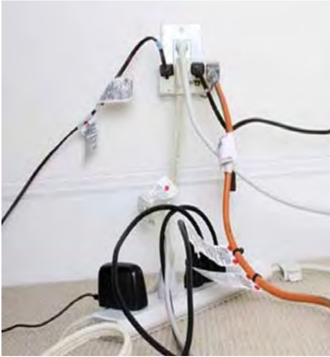
Figure 12: A single plug point with multiple chargers. No provision of sufficient plug points
