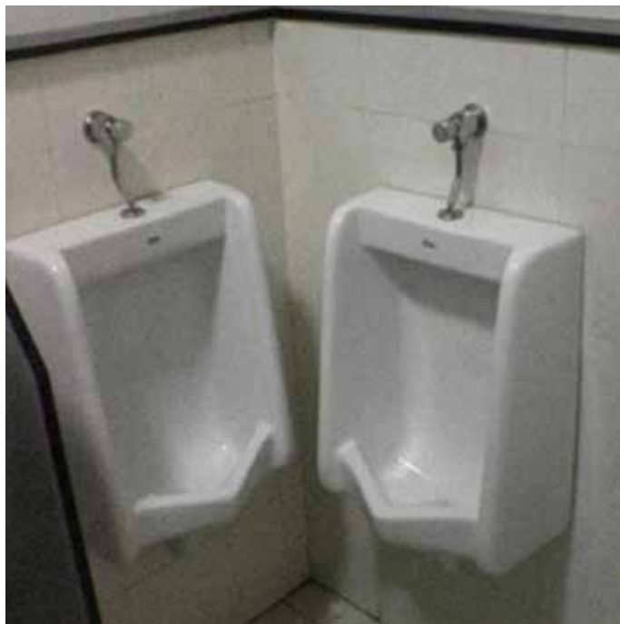
Figure 4: Side by side positioning of the urinals in public toilets without separator or usable space
