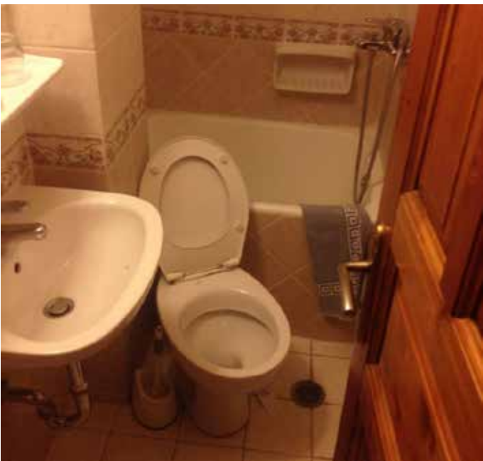
Figure 7: Corner WC with no space to stand, while close to the WHB
