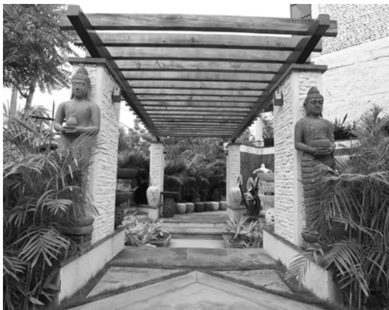
Cast in situ butch stones work on the pillars, with wooden trellis
