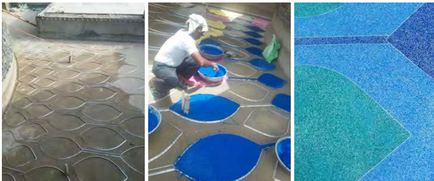
Cast in situ terrazzo in the water feature, using an innovative blend of colours and aggregates
